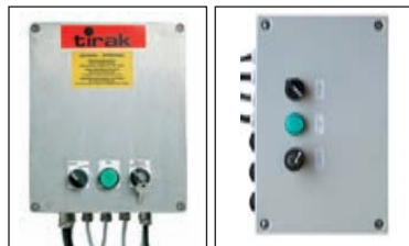
Fig. 9b Power cabinet X402 / L502 M500
